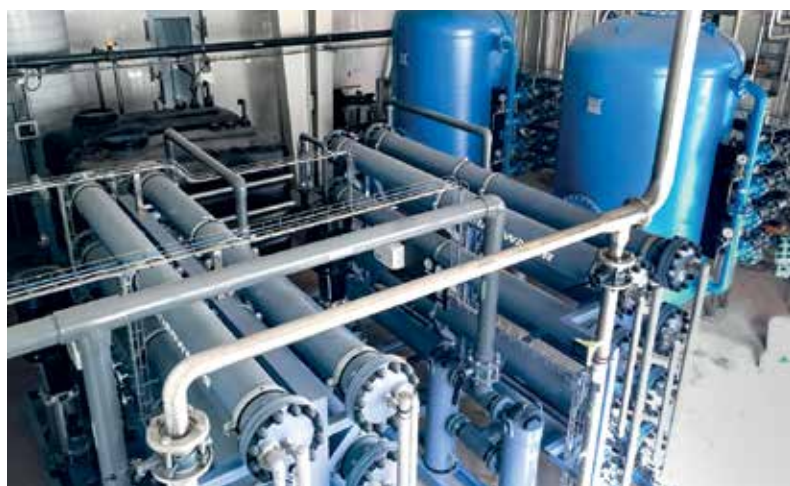
Complete water treatment solution based on pre-engineered EUROWATER units for RUD, Ukraine.
